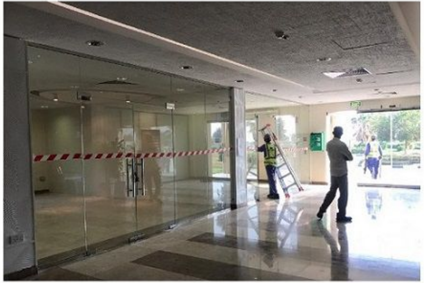
36. Project : Doha North Sewage Treatment Plant (DNSTP-Ummsalal) Scope : Office Glass Partitions and Glass Doors
