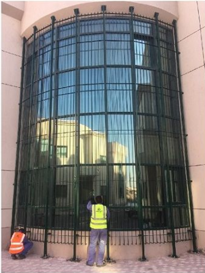
37. Project : Metal Works for Qatar Standards @ Mesaimeer Scope : Windows & Curtain Wall Grills
