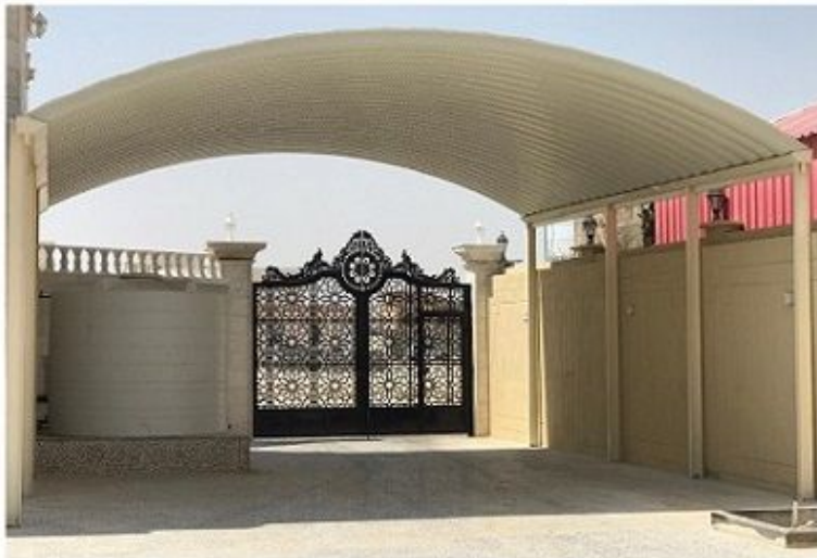
31. Project : Private Villa @ Saliya Scope : Decorative Steel gates and Kwik Span Car Park Shades
