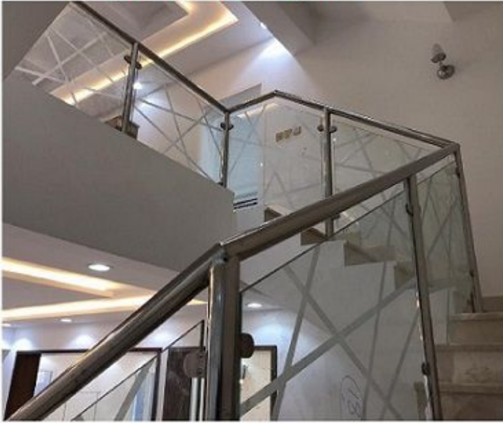
29. Project : Private Villa @ Al-Kheesa Scope : Stainless Steel Handrails with Sandblasted Glass Balustrades
