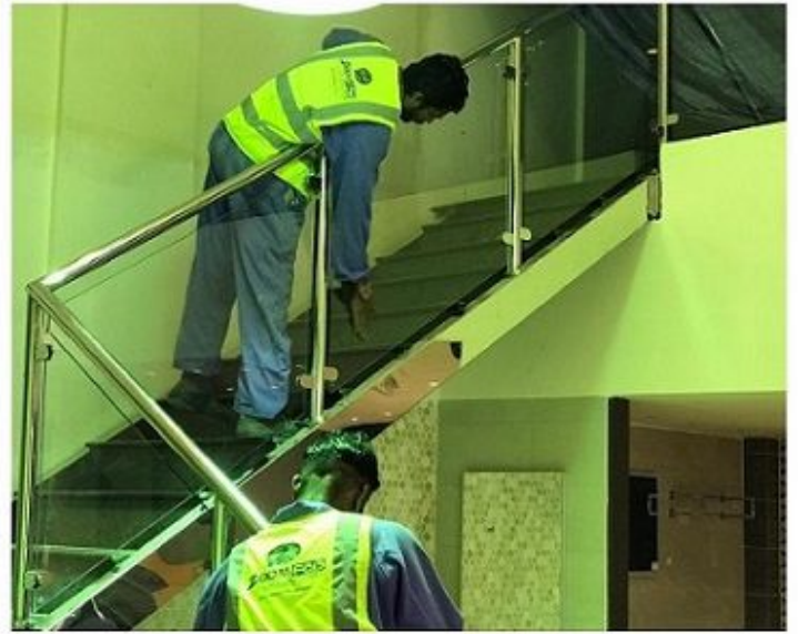
30. Project : Renovation of Office @ Salwa Road Scope : Steel Stair with SS Handrails and glass Balustrades
